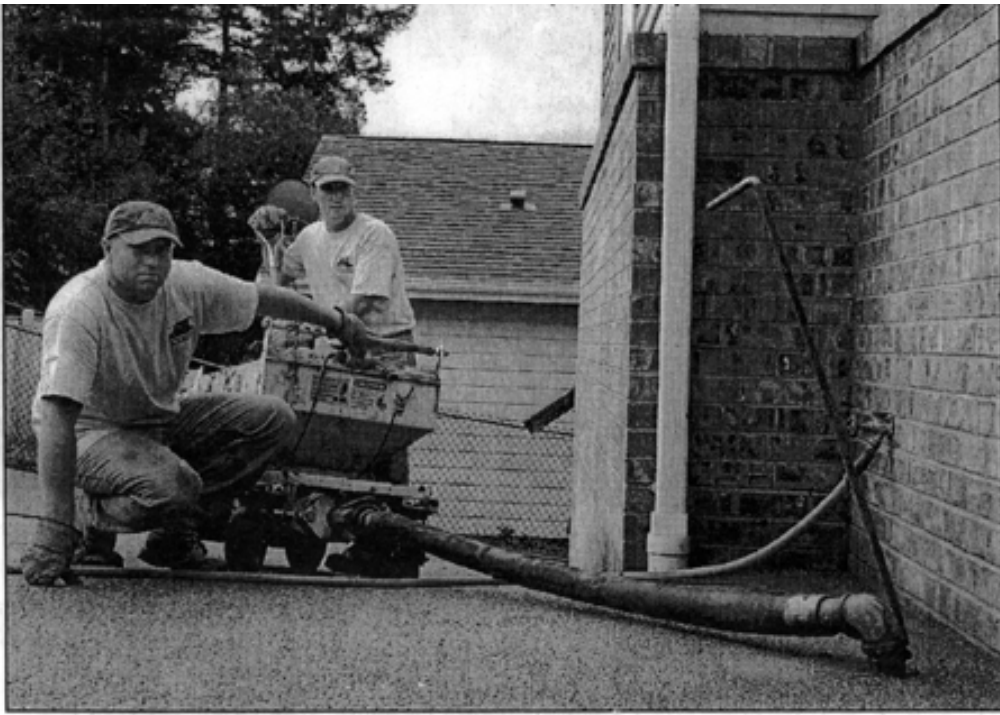
Super Slabjacking co-owners Ryan Earl (left) and Scott Schwehm watch as a cement mixture is pumped into one of several holes, drilled into a sinking concrete driveway on Camano Island. The process lifted the concrete surface back to its original height and eliminating a crack in the nearby brick façade. —NEWSphotos by John Dean
