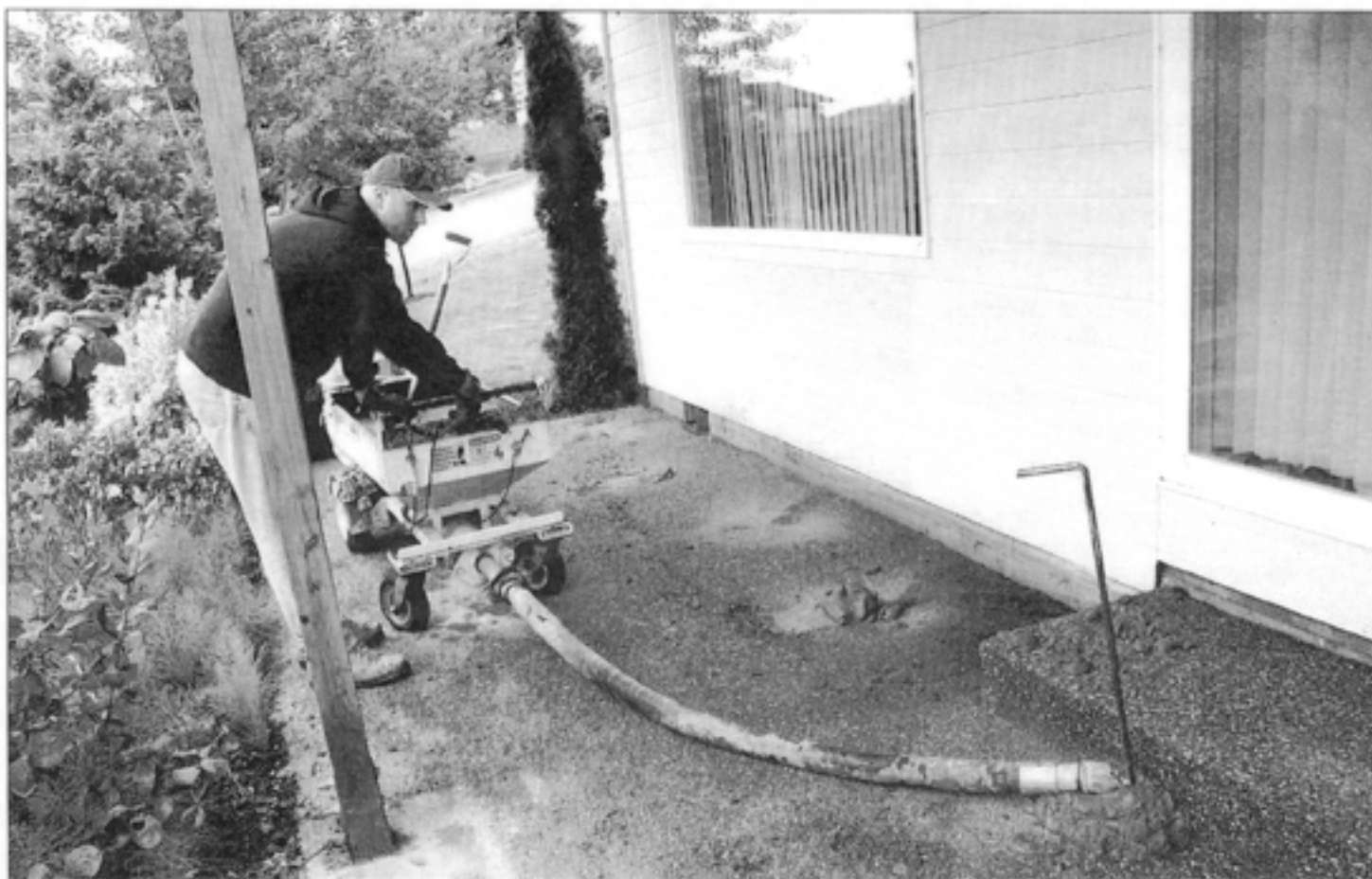
Ryan Earl of Superior Slabjacking pumps material underneath a concrete deck that needed to be raised approximately 6 inches.
