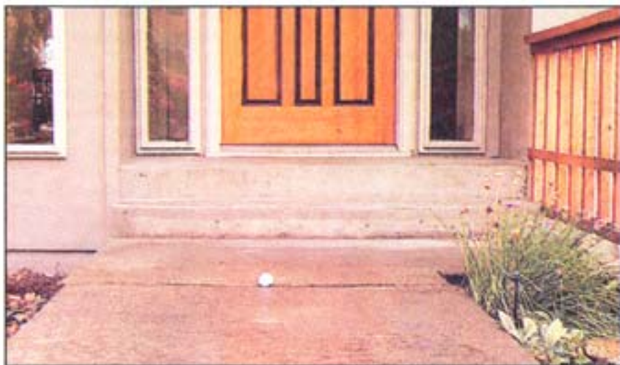
Photos courtesy of Superior Slabjacking Inc. "It is fascinating watching sunken concrete come up," said Patrick Hayes, vice president of sales and marketing for Superior Slabjacking Inc., which recently repaired this residential walkway, lifting the fallen concrete (at top) to make it level (above).
